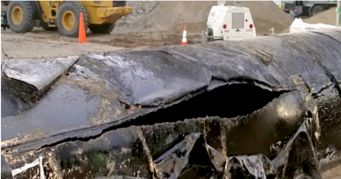
Image 1: Enbridge Line 6B Ruptured Pipeline 11
